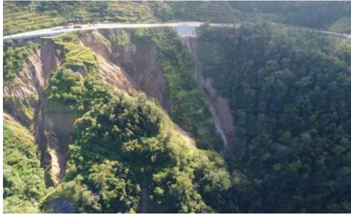
Landslide area at KM46, FT185 Simpang Pulai-Cameron Highlands Highway(captured on 24 February 2020)
