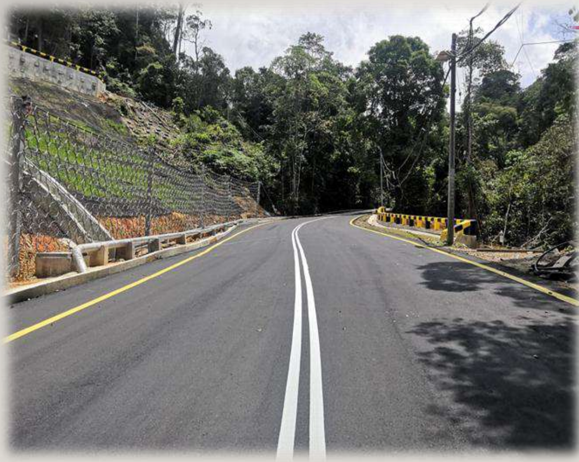
Rockfall Netting and Rock Fall Fencing
