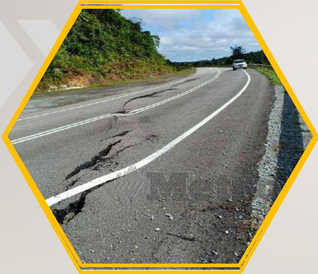
Tebing jalan retak/mendap/jatuh
